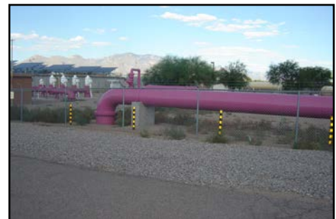
Purple irrigation pipes for treated effluent
