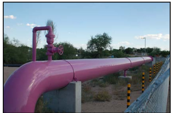
Reclaimed water distribution line
