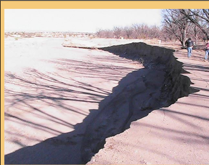
Photo # 28. Ground view of bank erosion w/in FICO.
