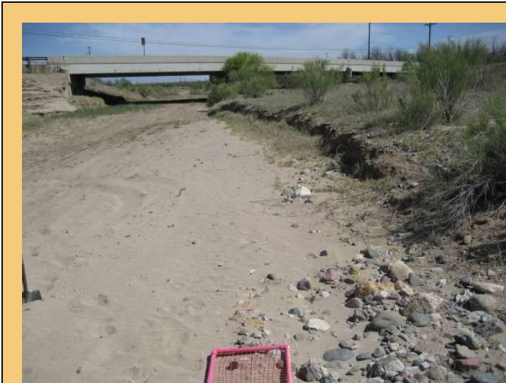
Photo #13. River channel near Sahuarita Road. View looking downstream toward the Sahuarita Rd. Bridge. Note that a high-flow terrace occupies the east 2/3 of the bridge.
