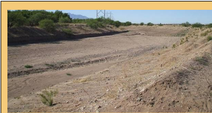
Photo #11. River channel between Pima Mine & Sahuarita Rds. View looking upstream mid-way between Pima Mine Road and Sahuarita Road.
